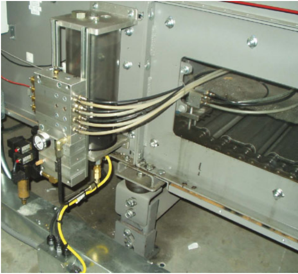
VSR system uses existing electrical controls.
